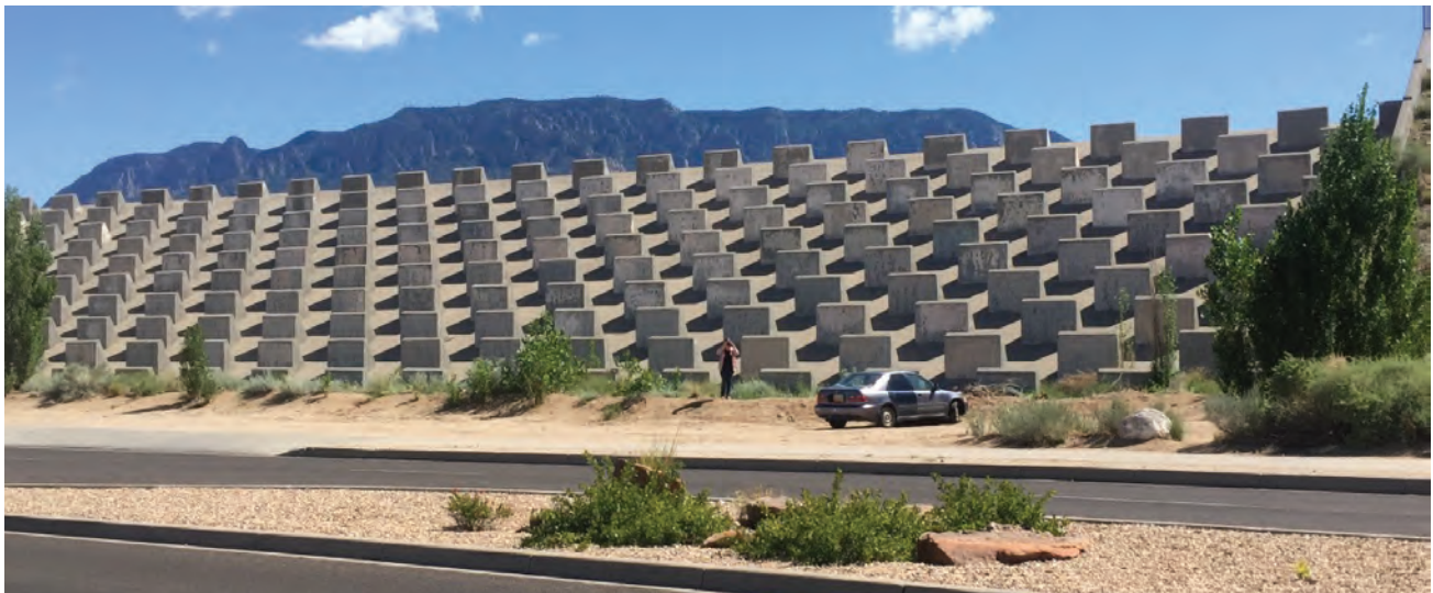
Figure 8.7. Photo of the emergency spillway for the John Robert dam owned by the Albuquerque Metropolitan Arroyo Flood Control Authority (AMAFCA). The spillway was designed to convey a flow of 23,600 cfs from a PMP storm. Photo by Bruce M. Thomson
